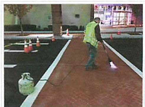
Construction of polymer cement overlay to change asphalt to brick texture and color to indicate high traffic crosswalk
